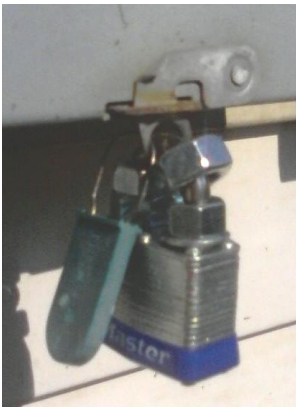
Pic. 2. Regular lock (be sure you get a SHACKLE lock) with nuts on front and back of lock loop. The plastic thing to the left of the lock is a tag the utility company puts thru the loop to make sure you do not open the box. Most meters never need fixing, so the tag has probably been there since at least the 1970s, if your house is that old. Hmm. Must mean analog meters work really well!
