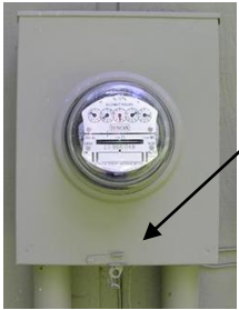
An electric box.
