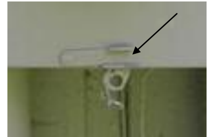
The loop on the electric box.
