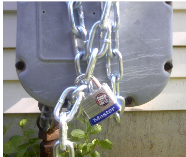
Close-up of lock on gas meter.
