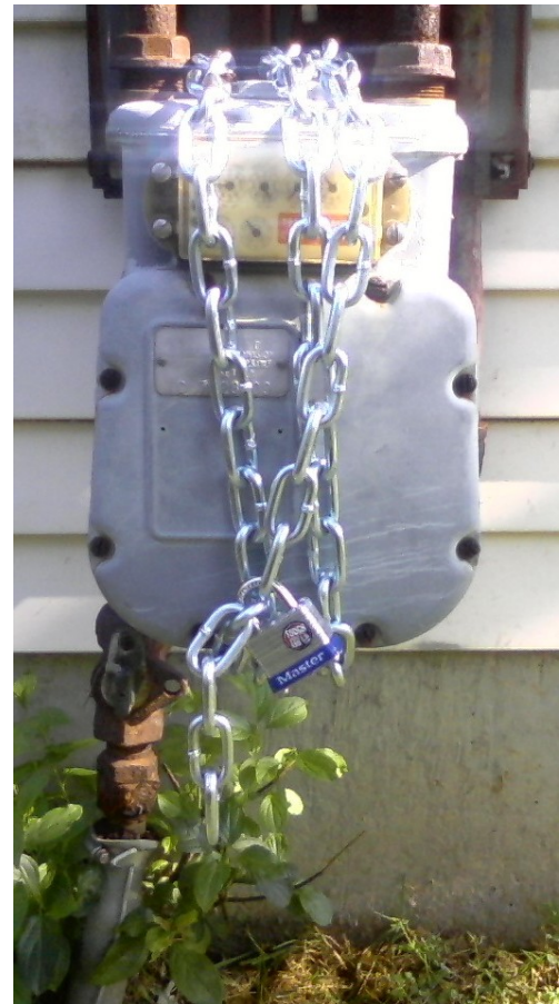
Gas meter. Note the meter at the top. Note the chain wrapped around three times and secured with a lock through two loops.
