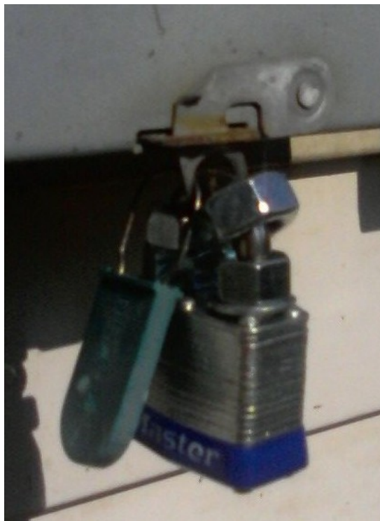
Pic 2. Regular lock with nuts on front and back of lock loop. The plastic thing in front of the lock is a thing the utility company puts thru the loop to make sure you do not open the box. Most meters never need fixing, so this loop has probably been there since at least the 1970s if your house is that old. Hmm. Must mean analog meters work really well!
